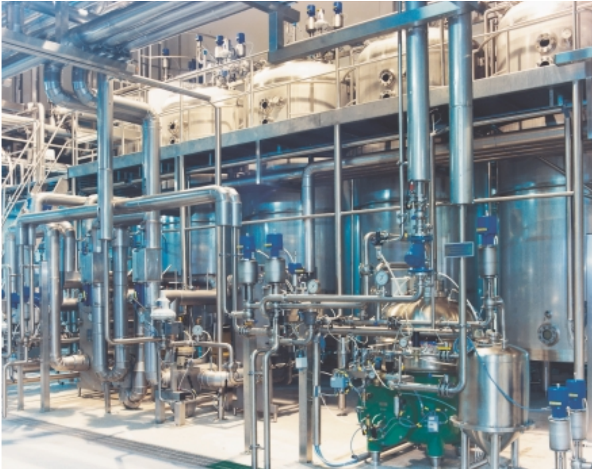
The Immocon process installed in the Sinebrychoff Brewery, Kerava, Finland.
